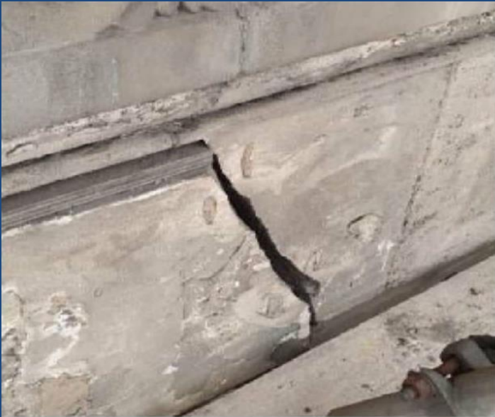
Cracked Stone Lintel (2021)
